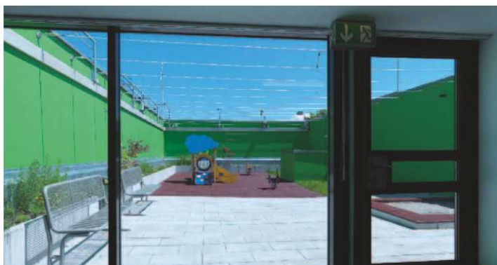
Emergency lighting leads the right way to safety and away from danger.
