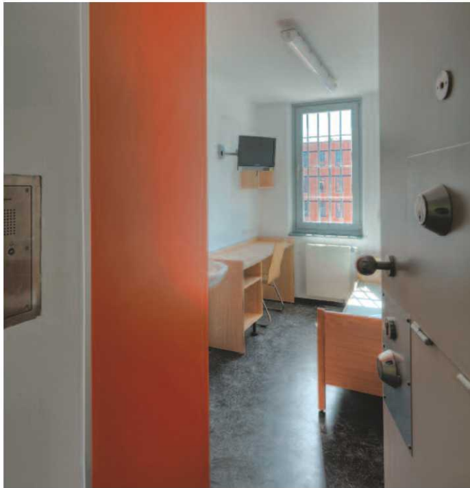
Prison cells are functionally optimized with the building management system GAMMA instabus .
